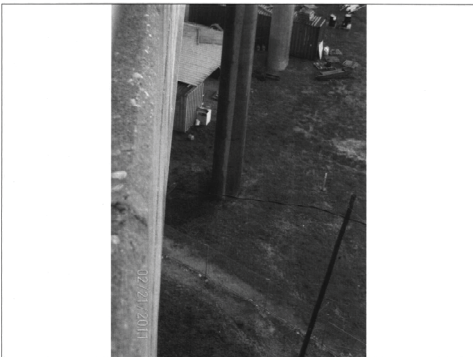
AI#:175084 Date: 2/21/2011 Description: Impacted Area
