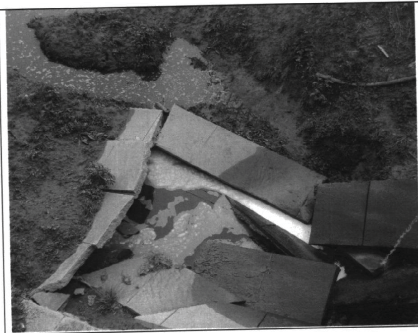
Photo #: 7 of 10 Time: 9:10 AM Description: Close-up of water as it leaves the pipe
