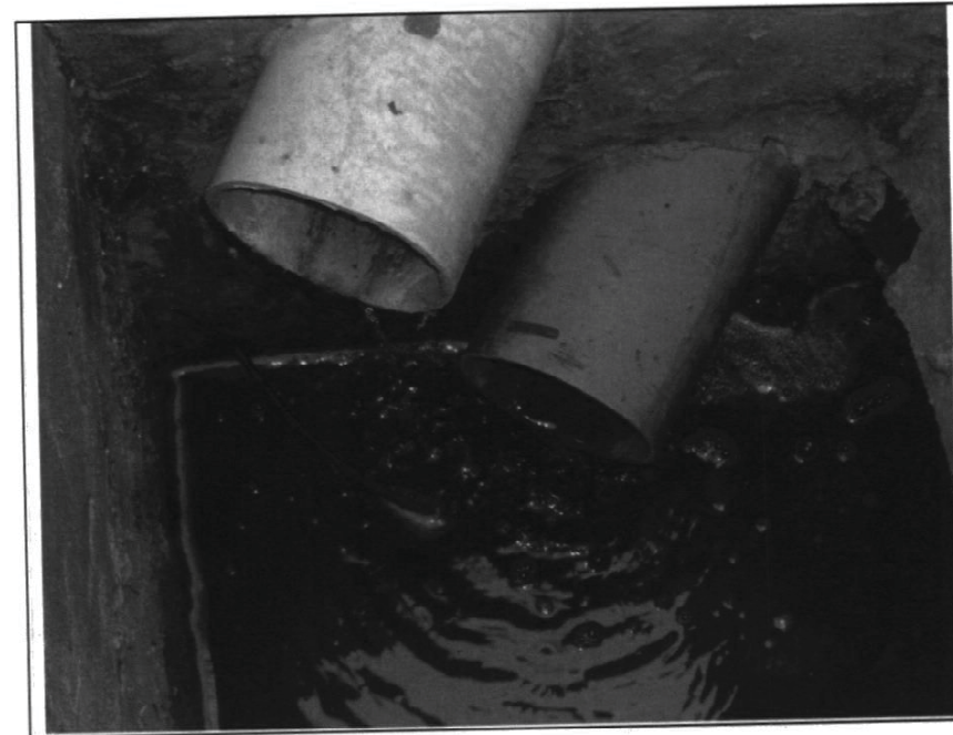
Photo #: 8 of 10 Time: 9:40 AM Description: Discharge pipes at Benny's Car Wash.
